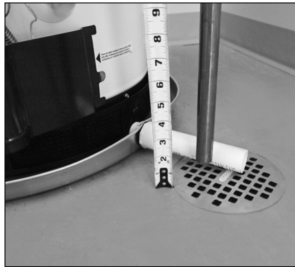
Figure 26 - Temperature and Pressure Relief Valve Pipe
